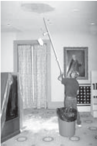
John Gardner, Old Capitol exhibits staff, removes weakened plaster from wet ceiling.
